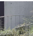
BAL-1 Steel Palisade Balustrade Paint Finish - protective coating Location: Level 5 + 6 balconies and rooftop terraces
